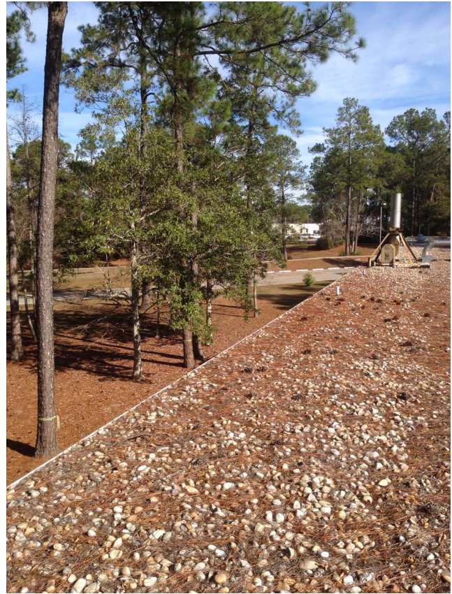
FIGURE 3.—Roof covered in debris.
